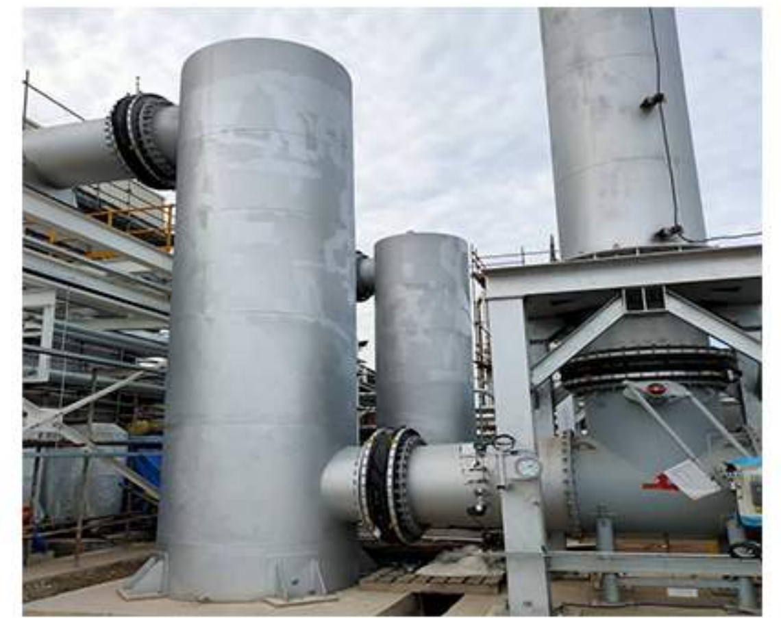
6MW Flue Gas Engine Silencer
