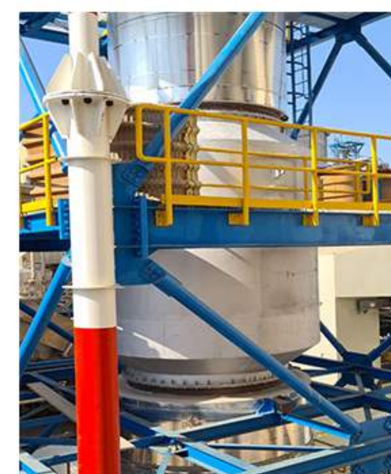
13MW Gas Turbine By-pass Stack Silencer
