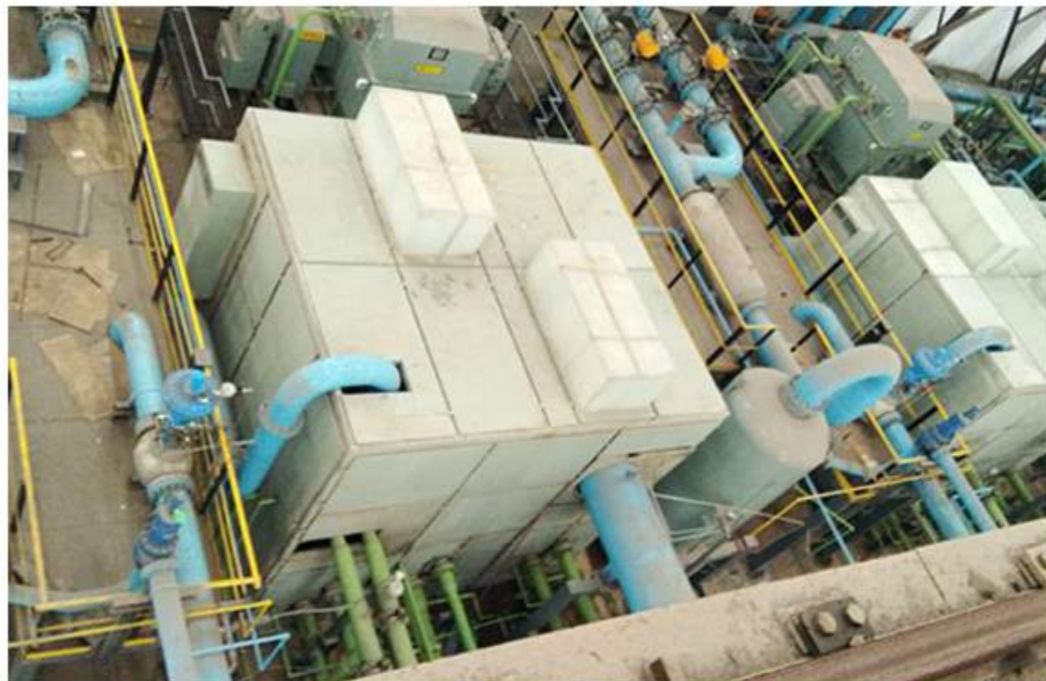
RINL-Viszag (compressor acoustic enclosure)
