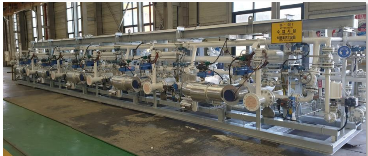
Valve Skid for Korean Gas plant Modeling & Fabrication
