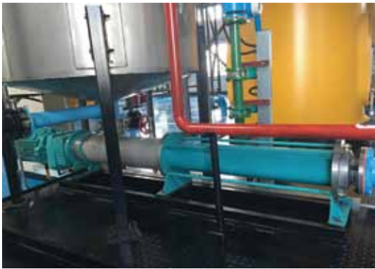
used to convey polymer solution
