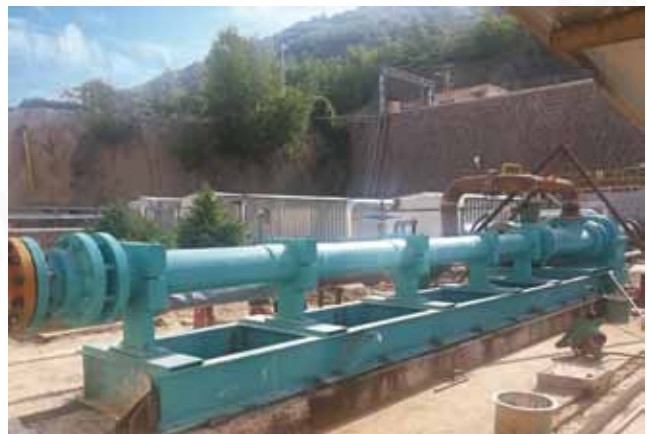
Pump to convey gas and oil mixture in Chinese western oil field
