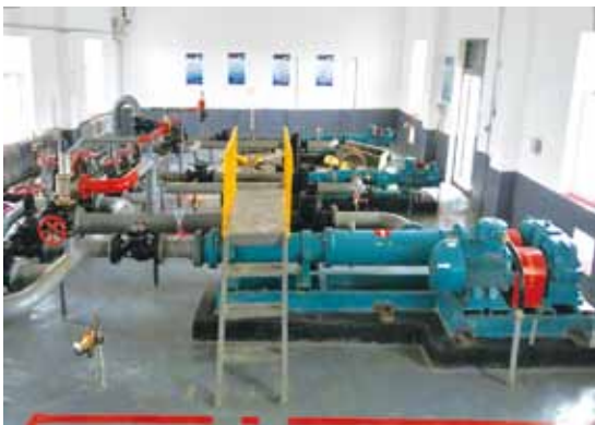
pump room in oil field
