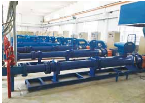
polymer configure station in oil field
