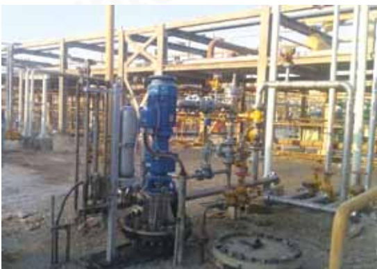
Vertical pump in Iran oil field
