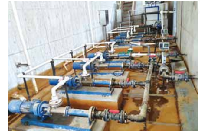
Additive injection pump
