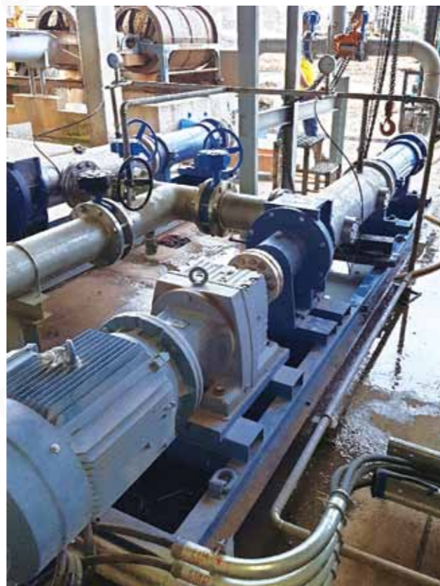
Subtor sludge conveyance pc pump
