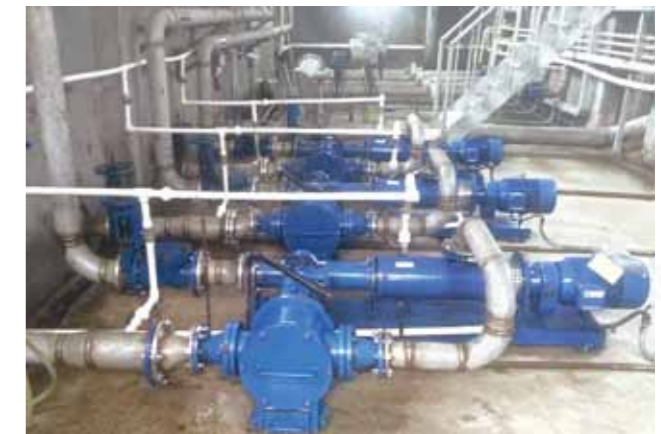
Macerator Installed before pump
