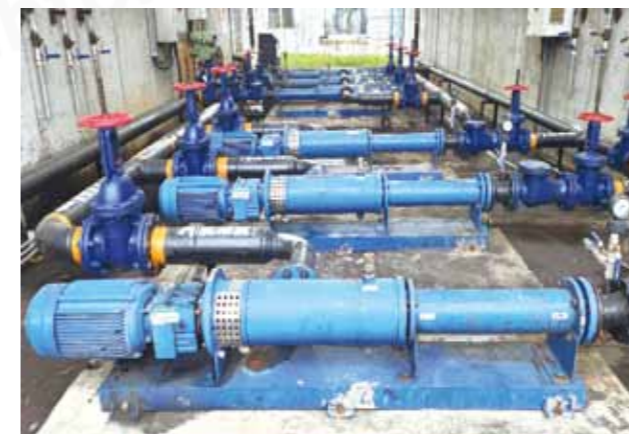
PC pump to transfer Sewage solid content 1-5%
